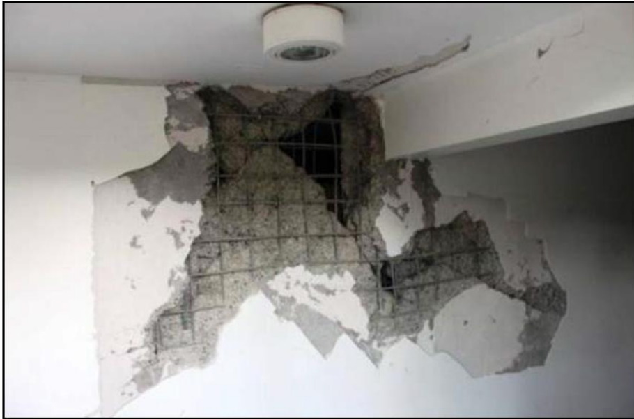
Figure 4-17 Damage observed in a solid wall panel below a stack of openings in the Torre Mayor building, Chillán (photo courtesy of EERI).
